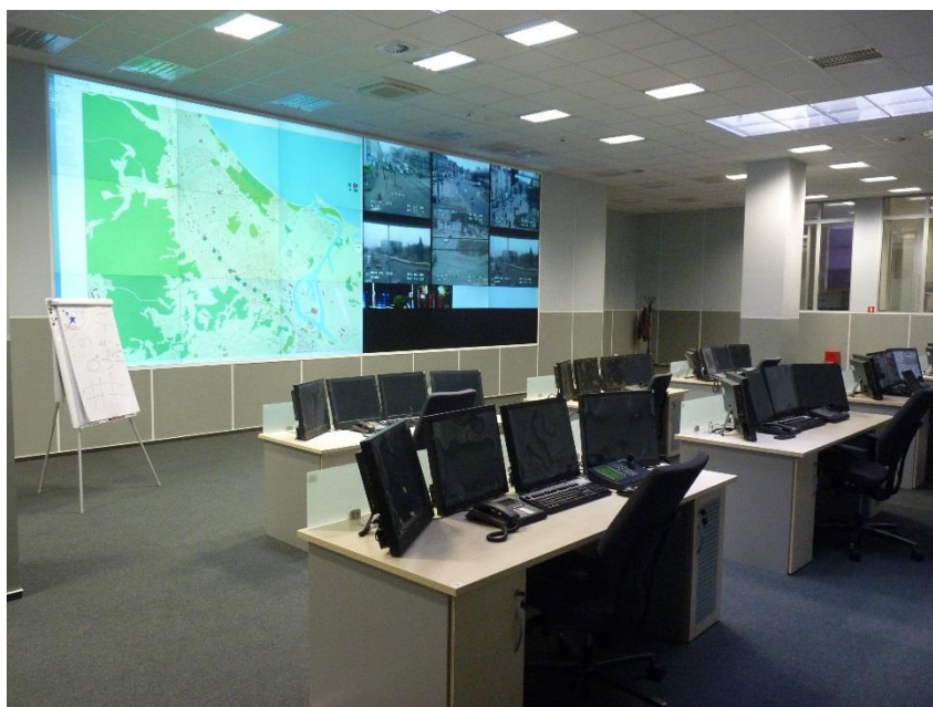
Figure 8: Tristar control room
